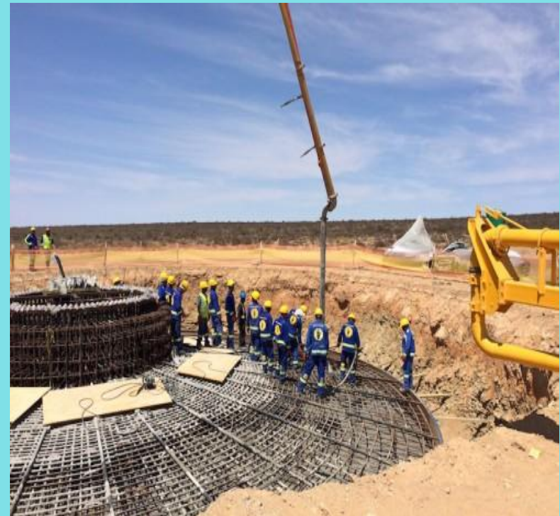
140 MW De Aar-2 North Wind
